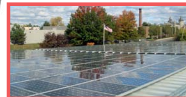
Lowell Regional Transit Authority Solar Array
